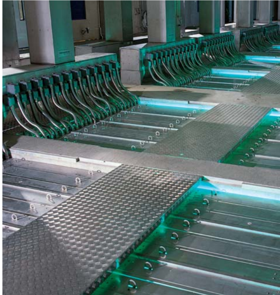
Worldwide largest UV system for waste water in Manukau, New Zealand. (Capacity: 14 m3/s)
