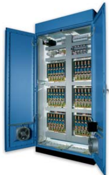
Arrangement of electronic ballasts inside an electrical cabinet
