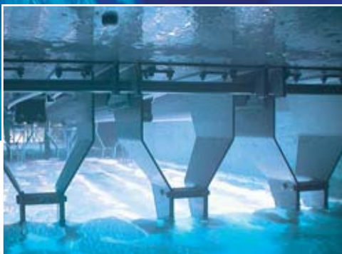
WEDECO System TAK 55: Waste water disinfection in Cassano Spinola / Italy.
