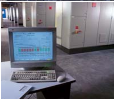
Supervision and maintenance via modem connection
